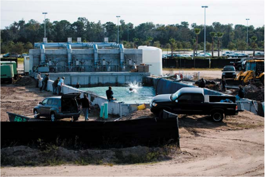
Fig. 6. The construction and preliminary use of a Surfpark. Photograph courtesy of Jimmy Wilson.
